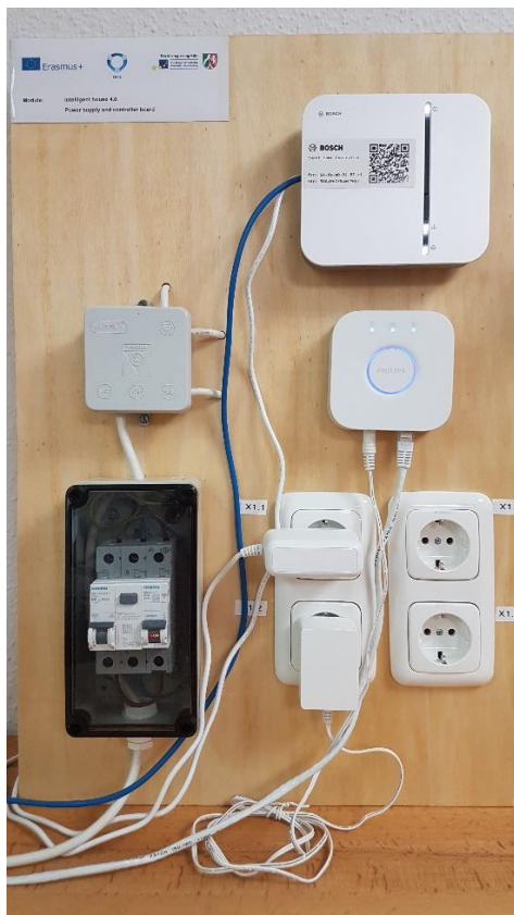
Module 1, Front With Bosch Smart Home Controller and Phillips Hue Controller
